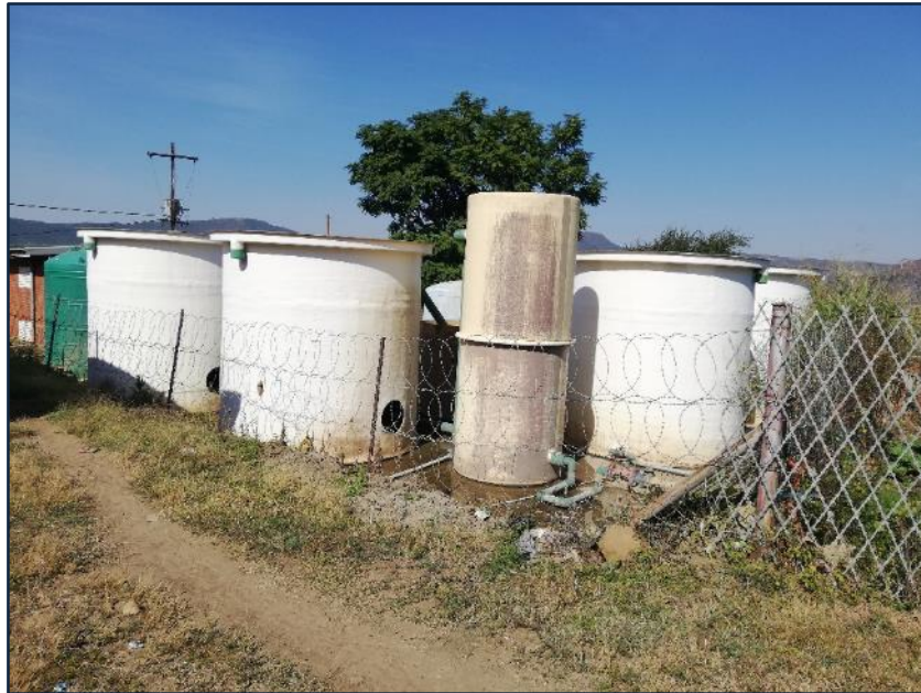
Figure 13.32 Tugela Estates WTP clarifiers (Umgeni Water 2019).
