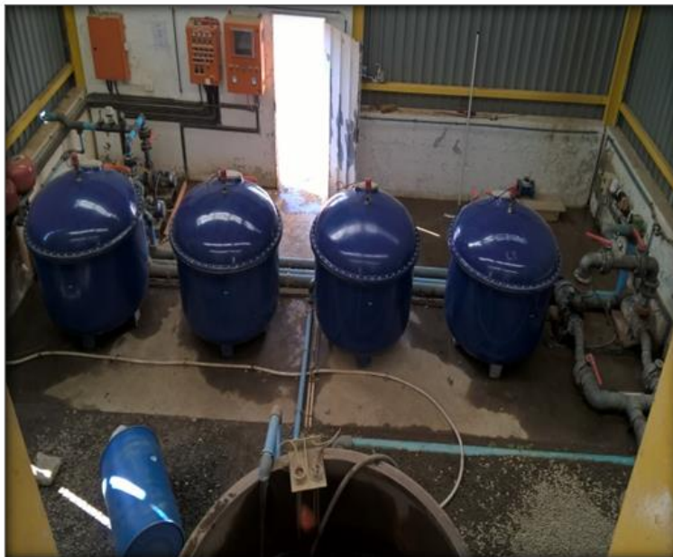
Figure 13.66 Weenen WTP (Umgeni Water 2017)
