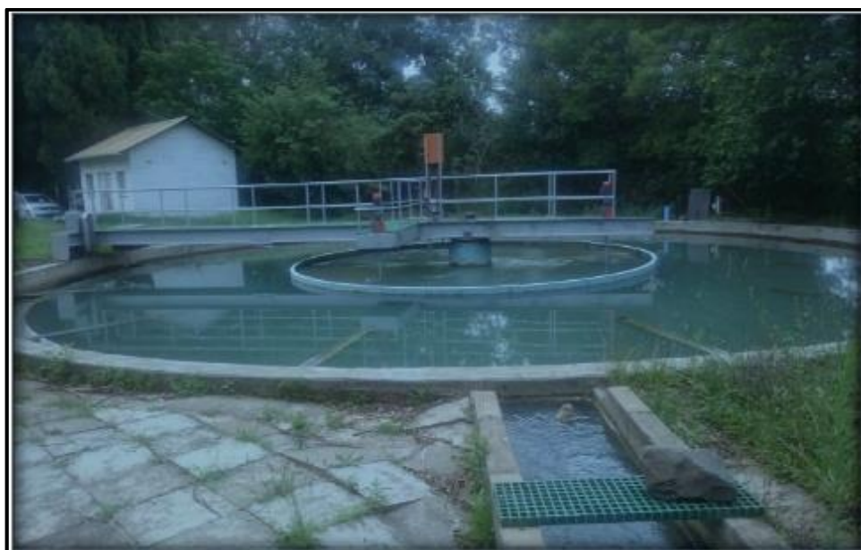
Figure 13.60 Archie Rodel WTP (Umgeni Water 2017)
