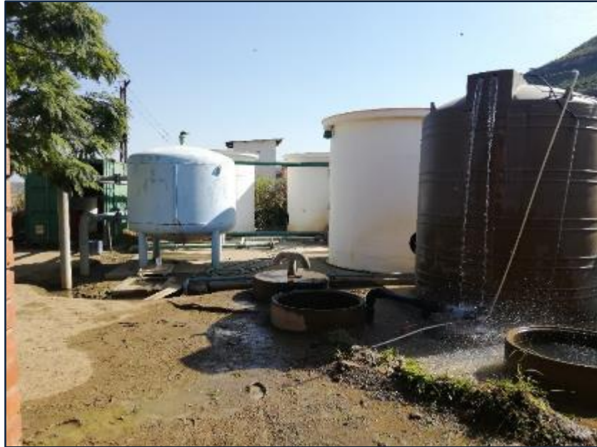
Figure 13.26 Tugela Estates Water Treatment Plant (Umgeni Water 2019).
