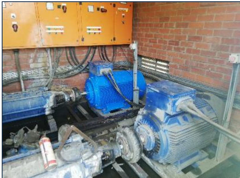
Figure 13.27 uMhlumayo Pump Station (Umgeni Water 2019).
