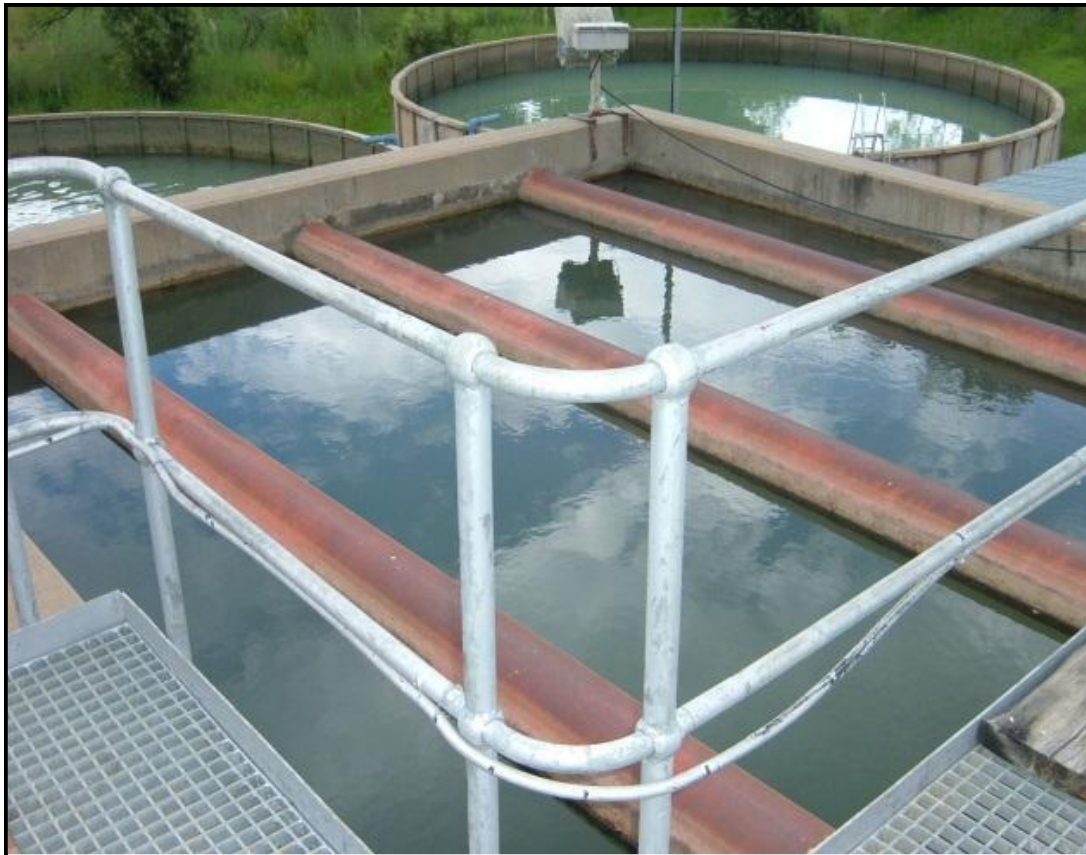
Figure 13.54 Colenso WTP (Umgeni Water 2017)
