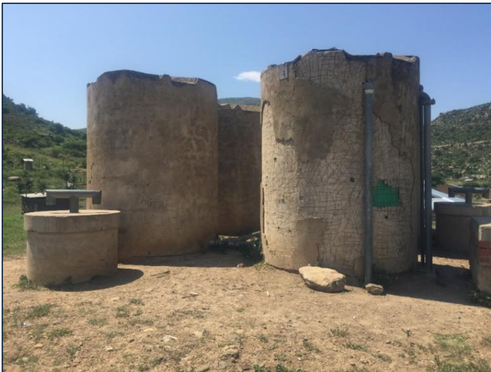
Figure 13.31 Tugela Estates Raw Water Holding Tanks (Umgeni Water 2019).
