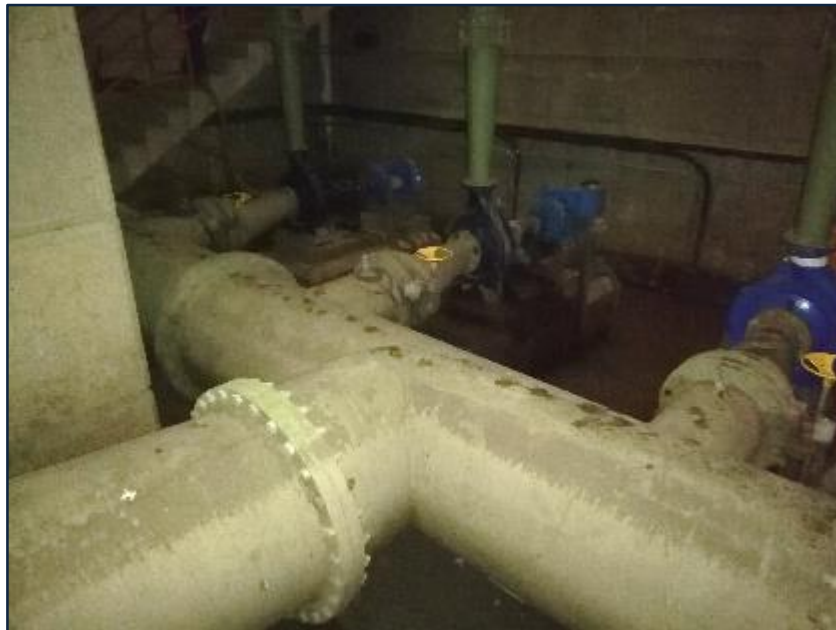
Figure 13.40 Olifantskop raw water pumps (Umgeni Water 2019).
