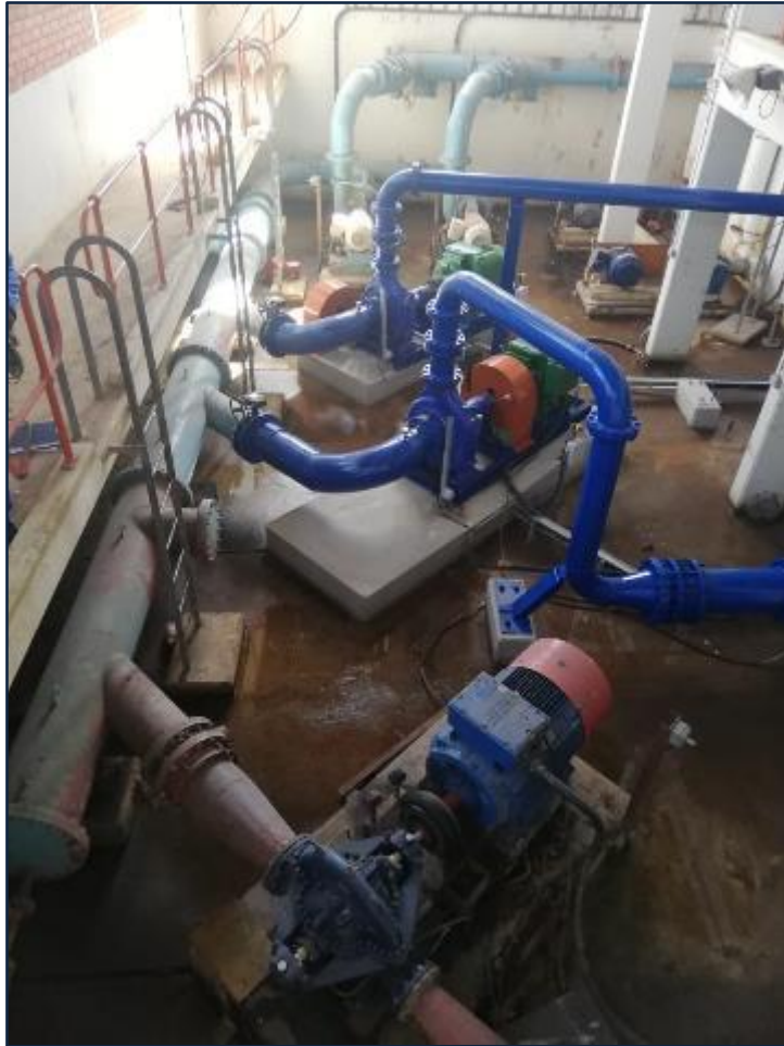
Figure 13.41 Olifantskop Clear Water Pump Station (Umgeni Water 2019).
