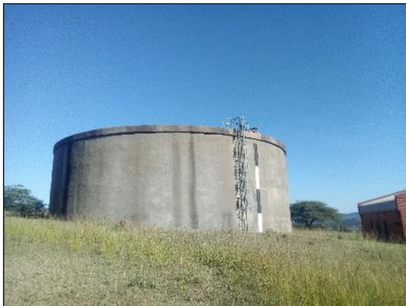
Figure 13.42 Petronella Reservoir (Umgeni Water 2019).
