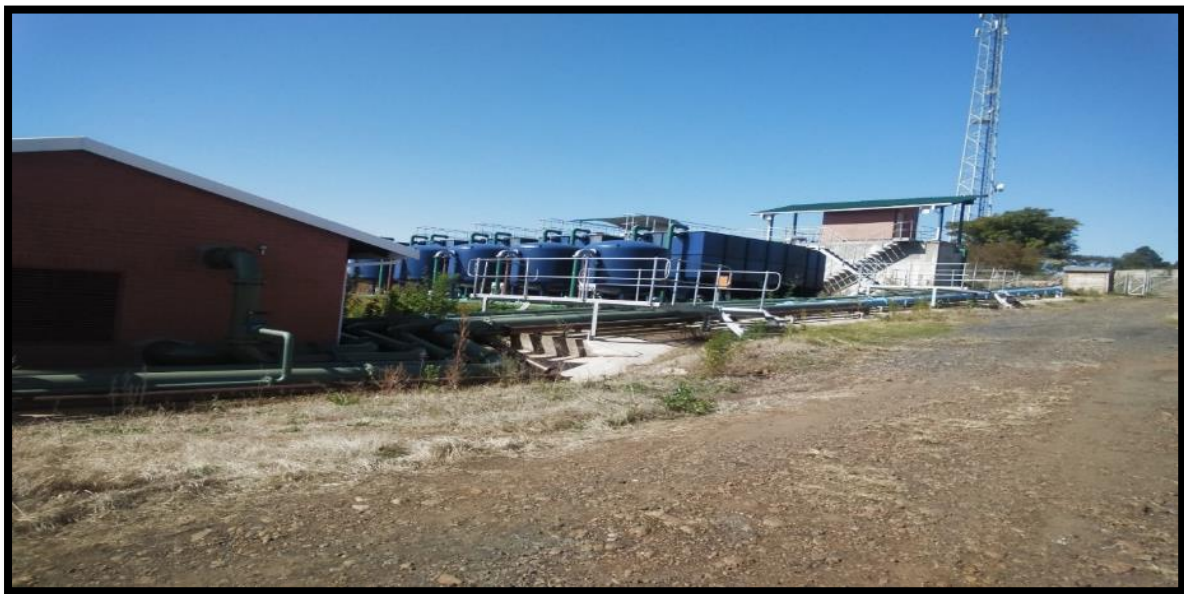
Figure 14.33 Photo of Durnacol Water Treatment Plant (May 2020).
