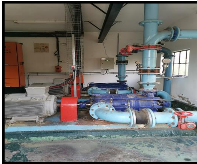
Figure 14.40 Utrecht Clear Water Pump Station
