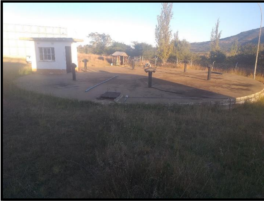
Figure 14.41 Utrecht Clear water Reservoir
