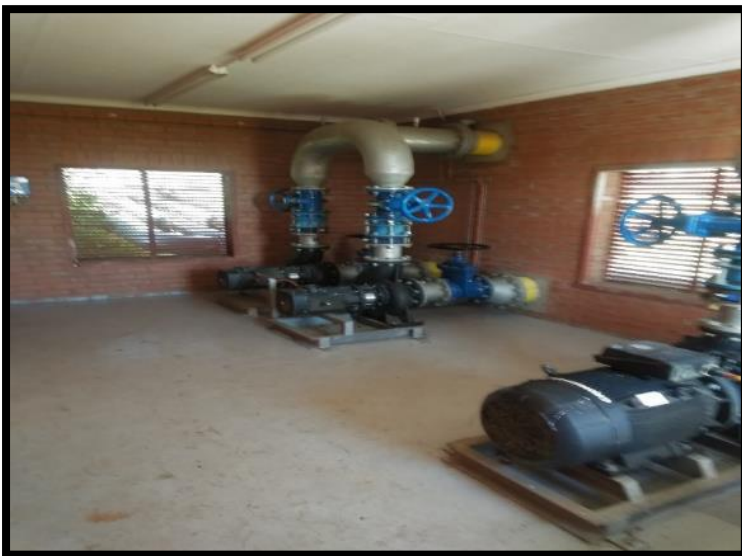
Figure 14.36 Durnacol Clear Water Pump Station (May 2020)
