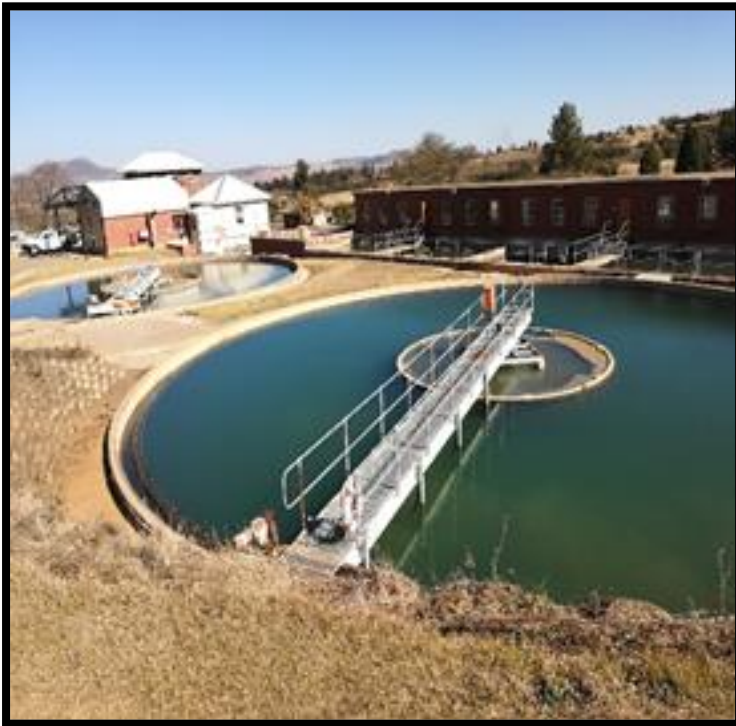
Figure 14.23 Photo of Biggarsberg WTP, Clarifiers (July 2019)
