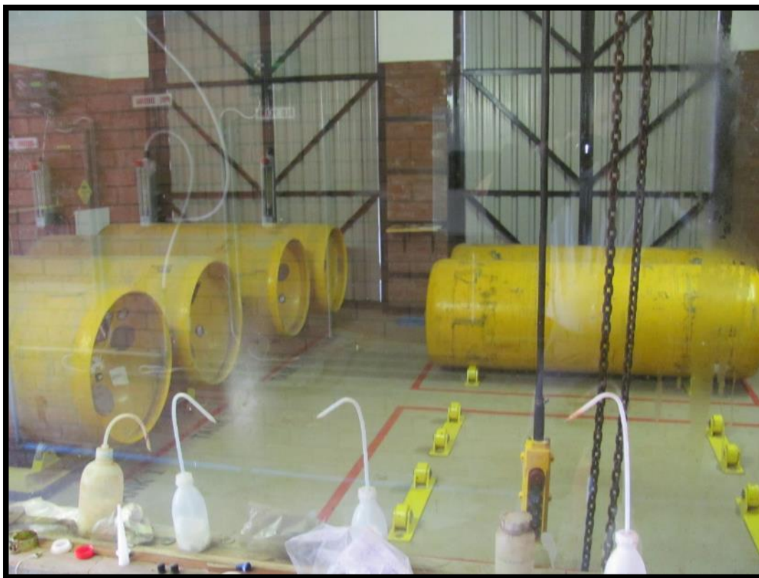
Figure 14.24 Photo of Chlorine Dosing Point at Biggarsberg WTP (July 2019)
