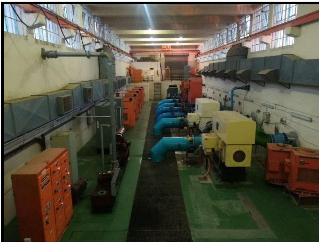
Figure 14.22 Photo of High Lift Pump Station at Ngagane WTP (May 2020)
