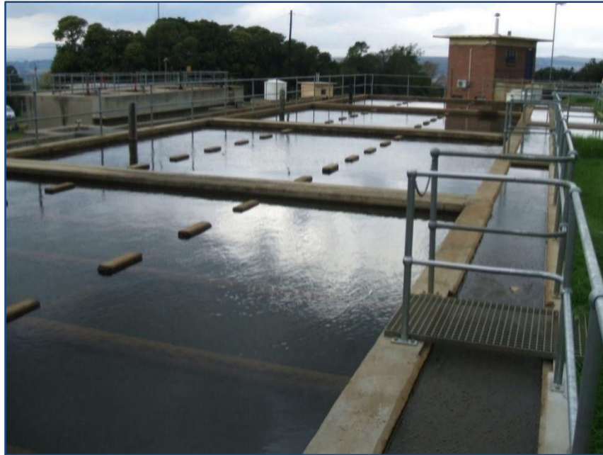
Figure 7.80 Mpofana WTP (uMgungundlovu District Municipality 2010).
