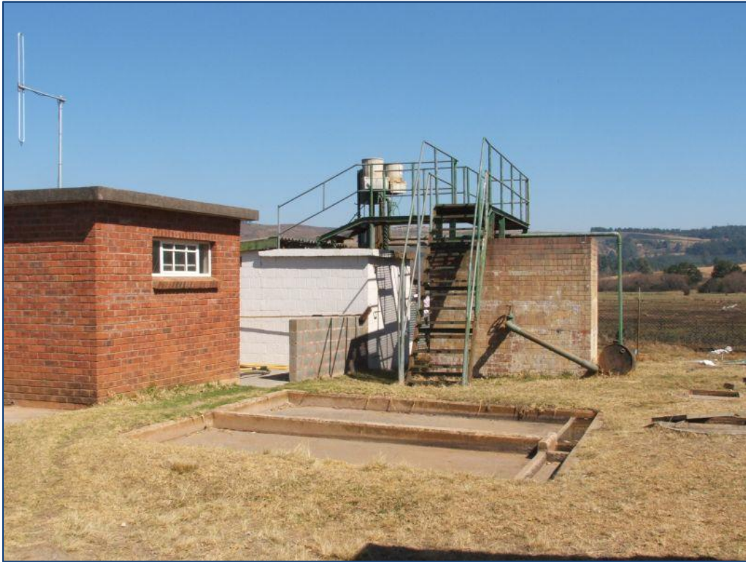
Figure 7.74 Lidgetton WTP sand wash bays with old dosing system (uMgungundlovu District Municipality 2010)
