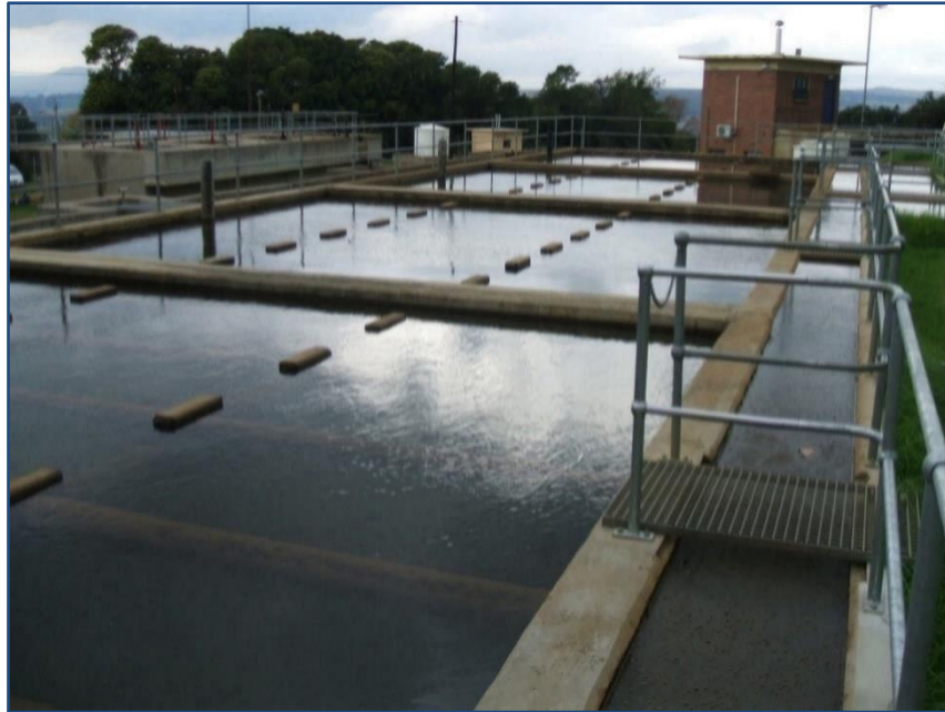
Figure 7.84 Mpofana WTP (uMgungundlovu District Municipality 2010).
