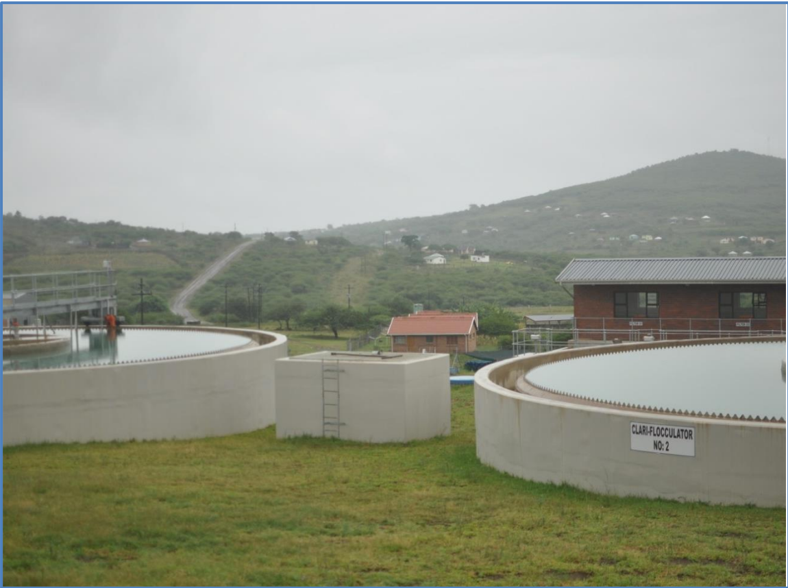
Figure 16.16 Photo of Middledrift WTP Clarifiers.
