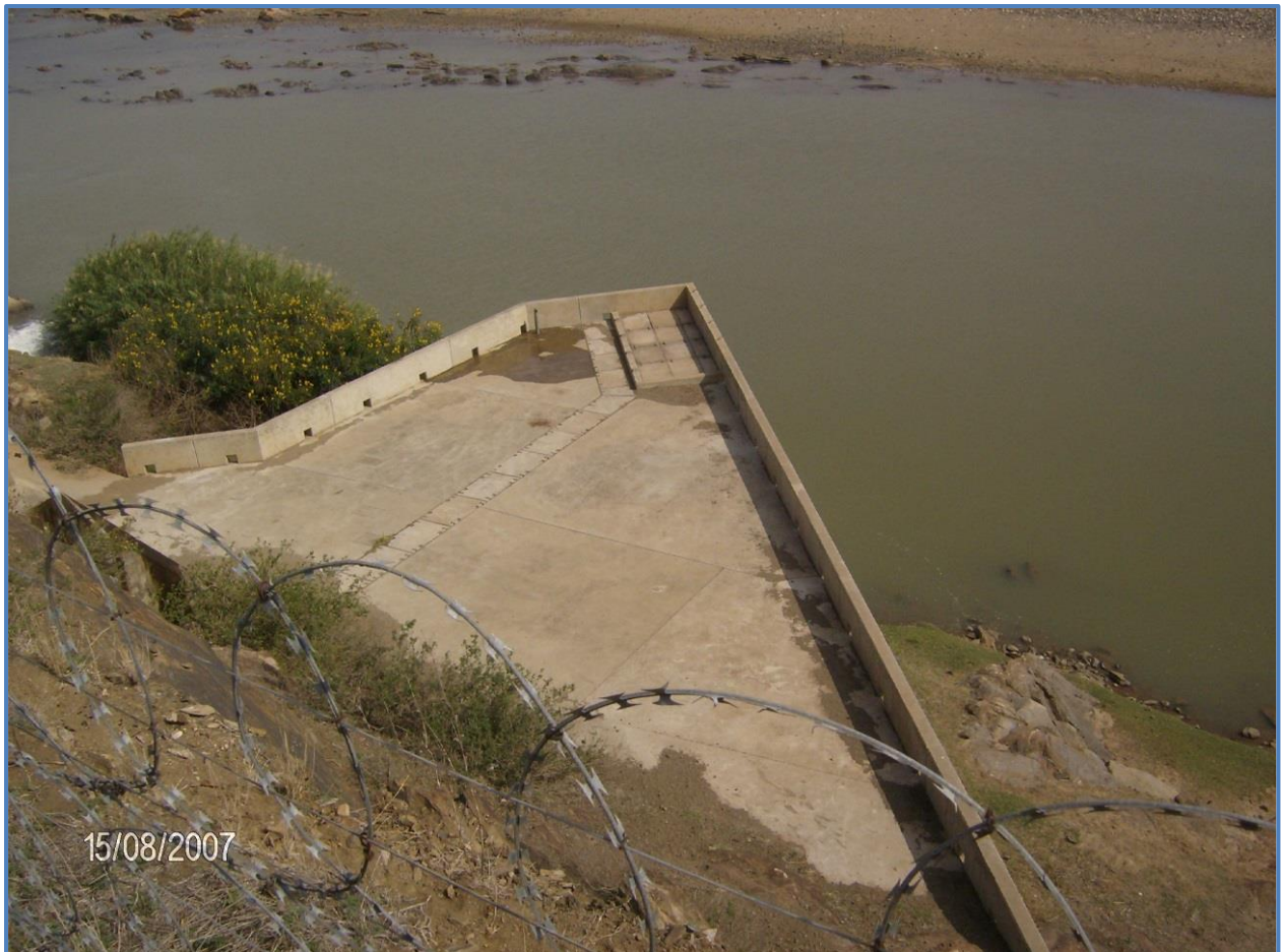
Figure 16.14 Thukela Transfer Scheme Abstraction Works.
